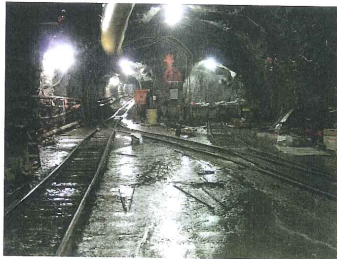
The team changed tunnel construction from a single drill and blast, double-high horseshoe tunnel for treated water pipes to excavation of two parallel single pipe TBM tunnels. CREDIT: Photo Courtesy of Schiavone/Picone
