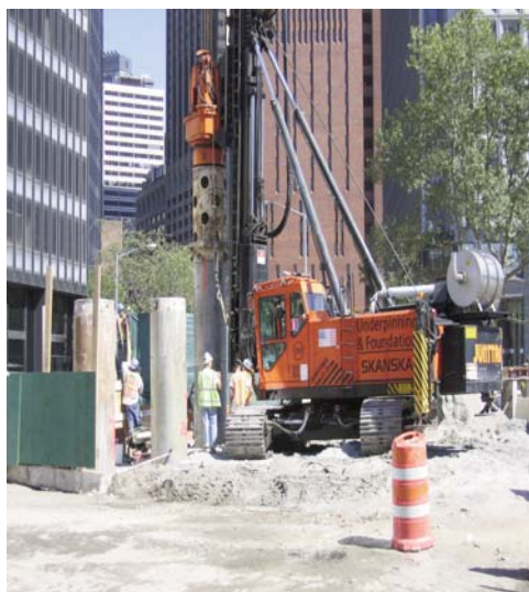
Subcontractor: Underpinning and Foundation installing secant piles at east wall of station
